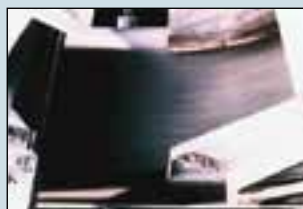
Coal stream discharging the spoon chute in the direction of belt travel at close to belt speed, minimising belt wear and spillage.
