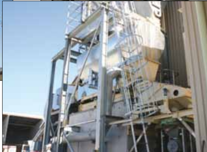
Sand drier: the processed sand is processed through the first of two sieves and a metal particle removal station prior to elevating and storage.
