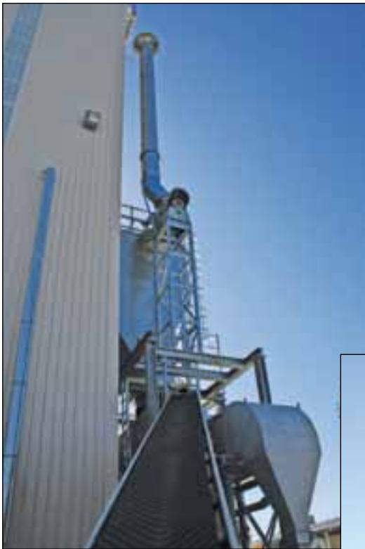
Sand load conveyor: wet sand is conveyed from the load hopper via incline conveyor to the fluid bed drier.
